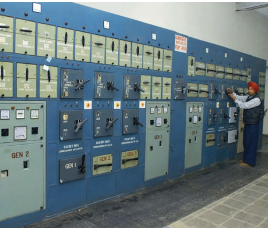
ABOVE: Electrical generator. The Dera provides generator backup in addition to other electrical services.
